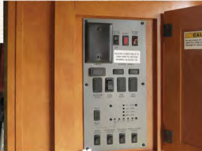
Central control panel with light and slide switches, tank monitors, awning, water heater and pump controls.
