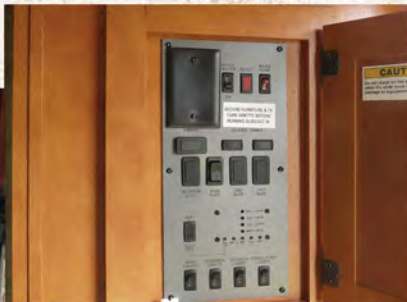
Central control panel with light and slide switches, tank monitors, awning, water heater and pump controls.
