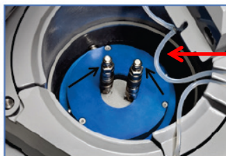
Figure 4, Generator Metal Caps
