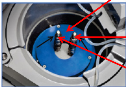
Figure 4, Generator Metal Caps
