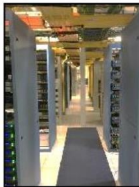
Interior Rack Spaces
