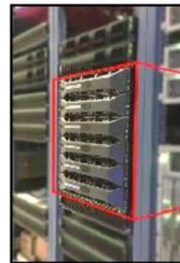
Google GGC Servers
