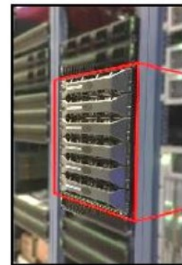
Google GGC Servers
