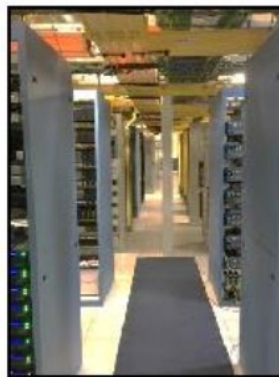
Interior Rack Spaces
