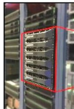
Google GGC Servers
