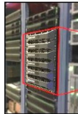
Google GGC Servers
