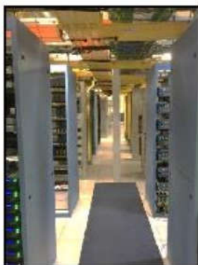
Interior Rack Spaces
