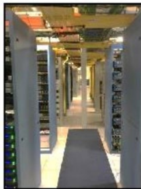
Interior Rack Spaces
