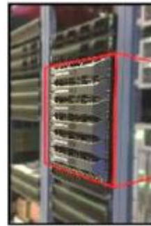
Google GGC Servers
