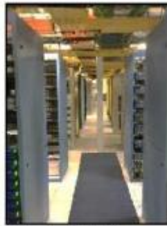
Interior Rack Spaces
