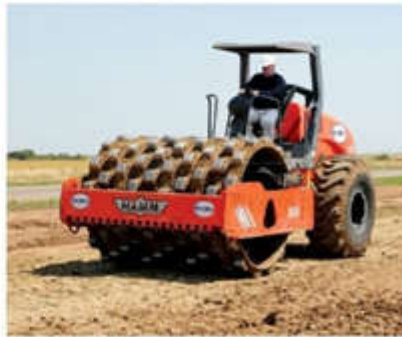
For earth compaction, Cornell Construction recently added a Hamm 100 horsepower MHP product roller that features an 80-inch drum and hydraulic steering. "It provides very good compaction," said Equipment Manager Gene Fiddly. "Our guys really like its maneuverability and production."
