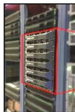
Google GGC Servers
