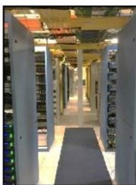
Interior Rack Spaces
