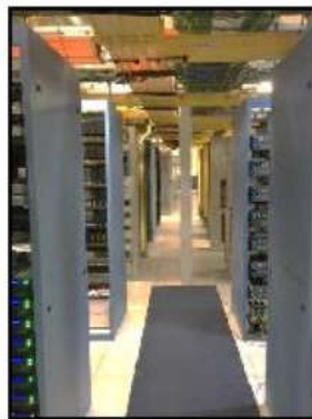
Interior Rack Spaces
