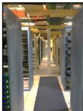
Interior Rack Spaces
