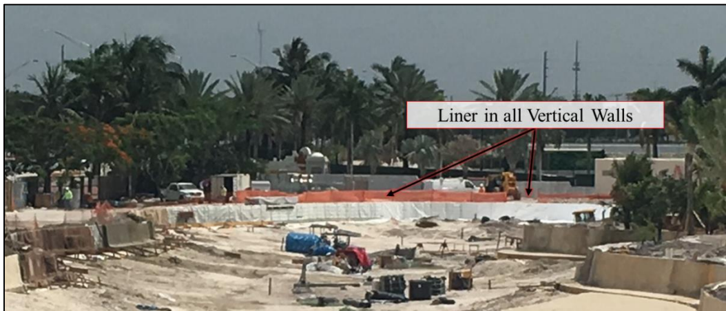
Figure 13: Lagoon during construction showing liner in vertical walls, where all the vertical walls were covered with a plastic liner
