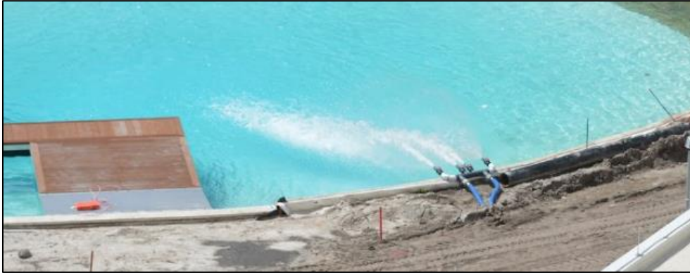
Figure 11: Fresh water feeding pipes
