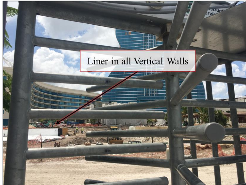
Figure 14: Lagoon during construction showing liner in vertical walls, where all the vertical walls were covered with a plastic liner
