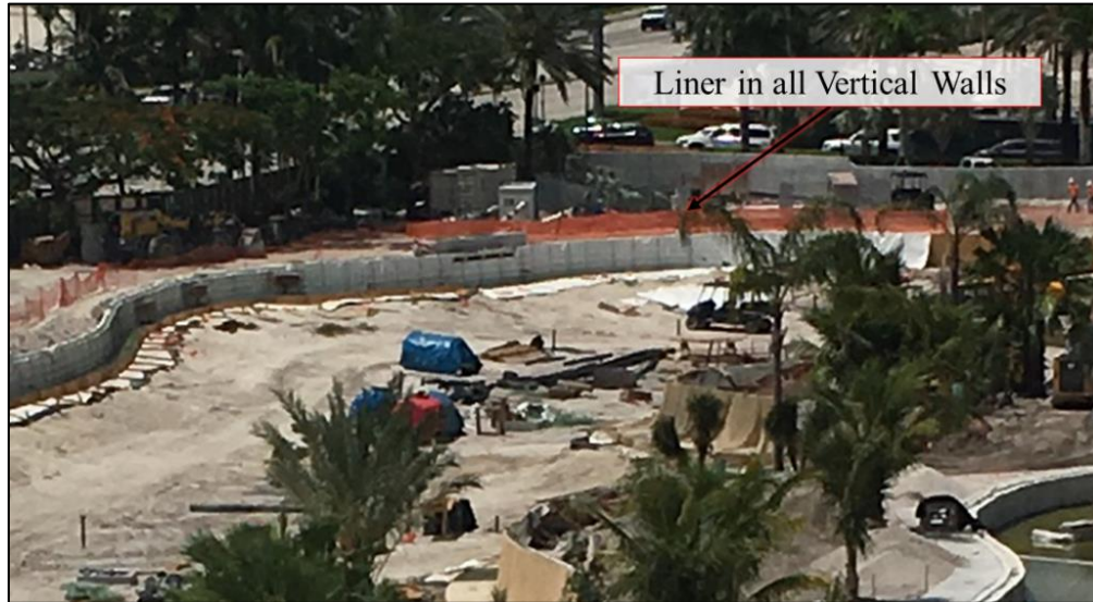
Figure 12: Lagoon during construction showing liner in the vertical walls, where all the vertical walls were covered with a plastic liner
