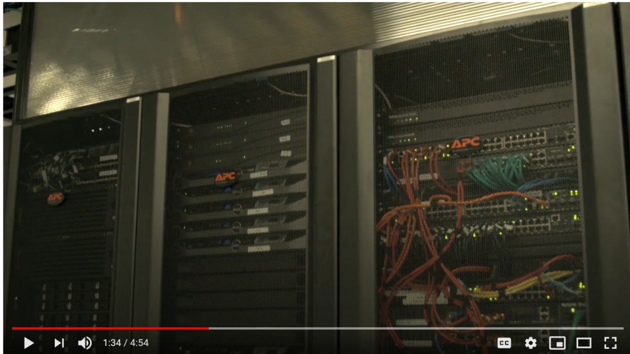
Green House Data - Cheyenne 2 Data Center Facility
