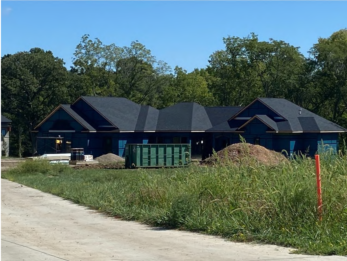
Photograph of Home Using WeatherLogic Panels and WeatherLogic Tape in Des Moines, Iowa Taken in September 2021
