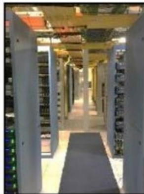
Interior Rack Spaces
