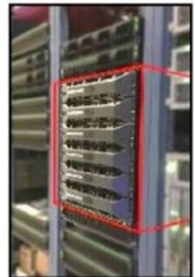
Google GGC Servers
