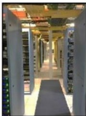
Interior Rack Spaces
